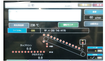
Heat Treatment Temperature Displayed
